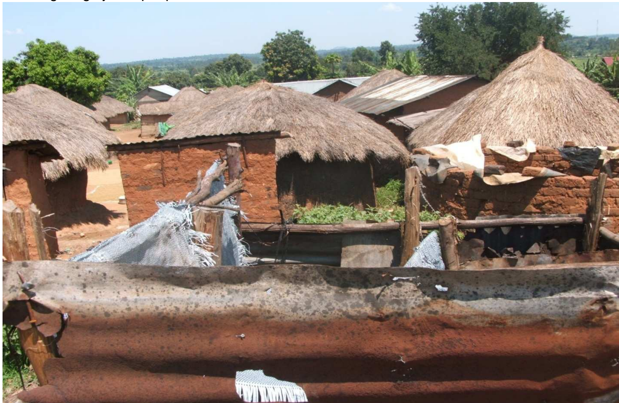
Figure 1 Poor quality housing and overcrowding
